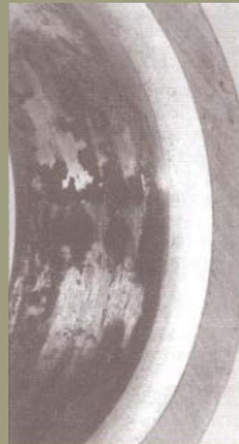
Widespread development of contact rust in the hole of an adjustable ball bearing.
